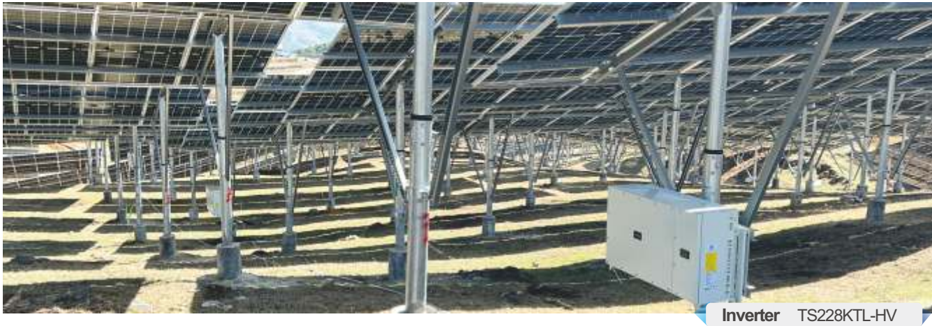
Yunnan Qiaojia 240MW Photovoltaic Power Plant
