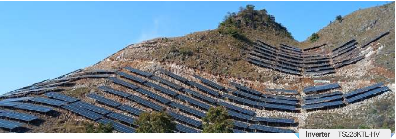
Guizhou Yingshan 120MW Photovoltaic Power Plant
