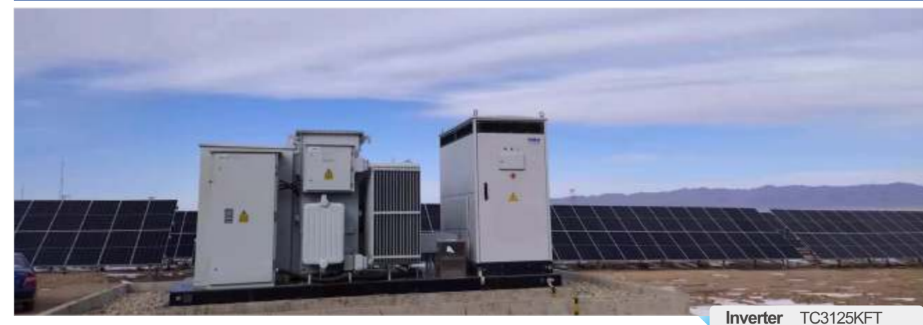
Gansu Yumen Oilfield 200MW Photovoltaic Power Plant
