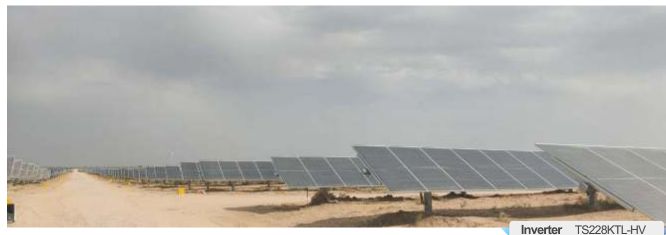
India Adani 50MW Photovoltaic Power Plant
