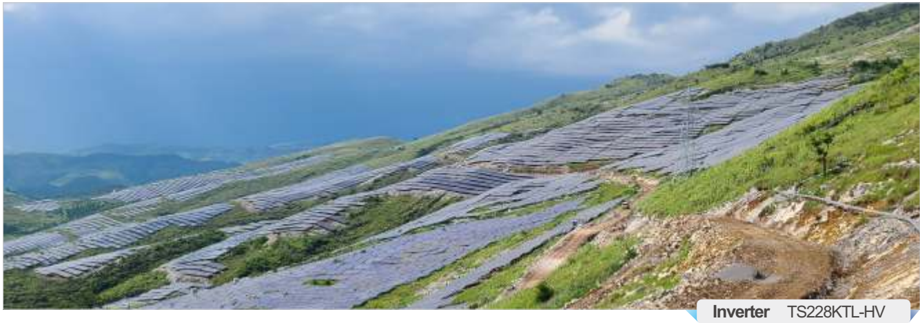
Guizhou Guanling 100MW Photovoltaic Power Plant
